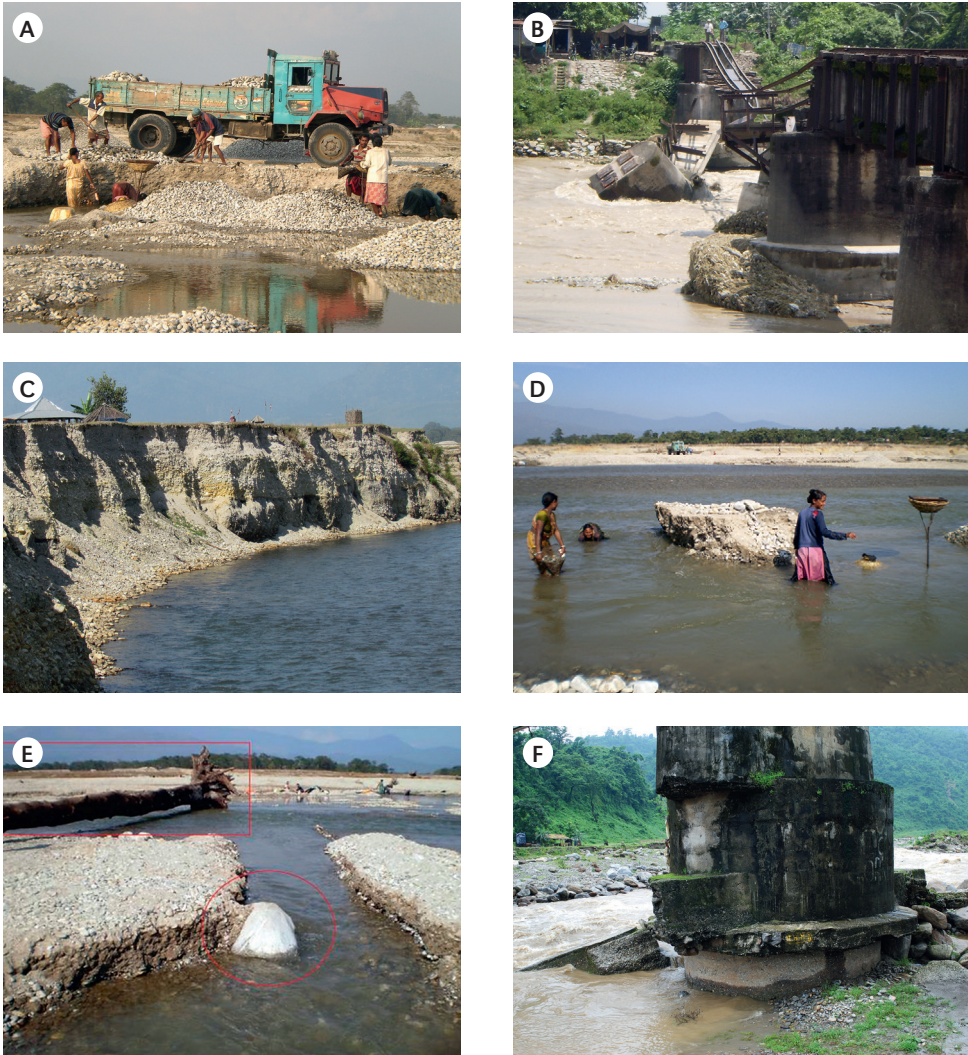
Figure 2. A – Bed material extraction from the riverbed in segment II; B – Damage of Railway Bridge downstream of N.H 31, in 2009; C – Exposed retreating banks upstream of N.H 31; D – Extraction of bar deposits upstream of N.H 31; E – Tree trunk and big boulder exposed due to bed incision at extraction site of segment II; F – Bridge pier at upper piedmont segment along the lower Balason River
