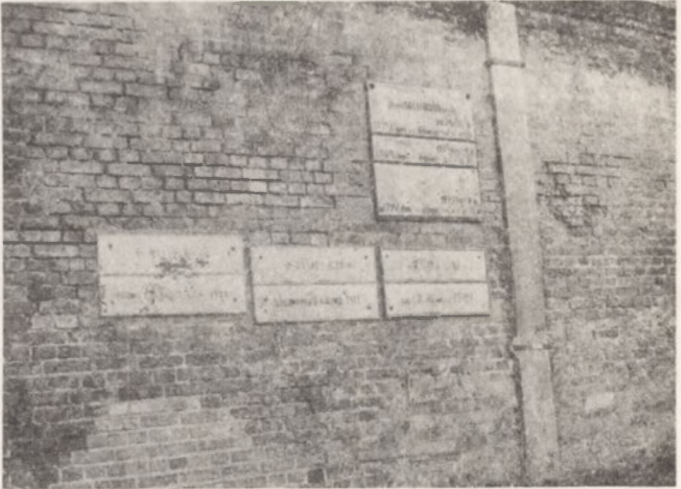
Photo 1. The marks of flood water levels during breakup period on the old town wall in Toruń
