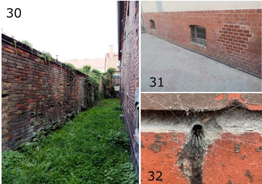
Figs 30–32. Site of occurrence of Segestria bavarica : 30 – Eroding brick walls (photo HS), 31 – Cracks in the external walls of buildings (photo DMS), 32 – Nests of S. bavarica in the walls (photo HB).
