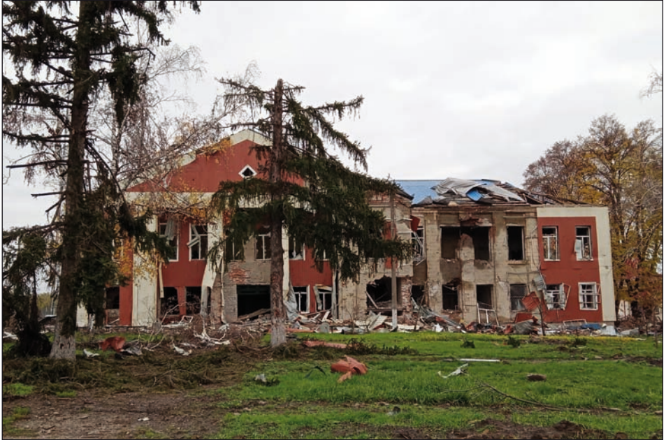
Destroyed building from the beginning of the 20 th century in the village of Drobisheve, Donetsk Oblast. Photo by Dmytro Klochko
