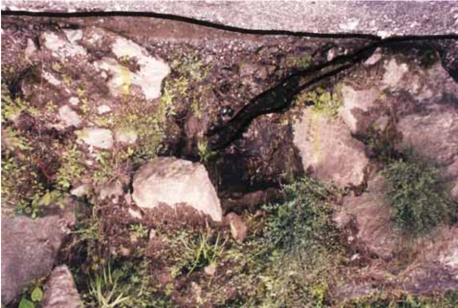
Figure 4. Visible cracks and fissures facilitate the piping and deep drainage
