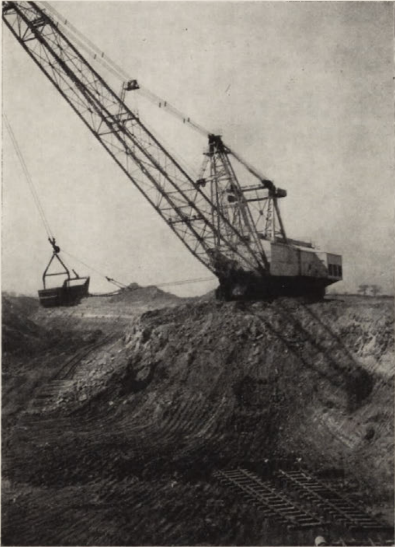
Fig. 2. An "opencast" ironstone quarry ("Type 2") in Northamptonshire Large "walking dragline" excavates overburden, creating "hill-and-dale" spoil heaps
