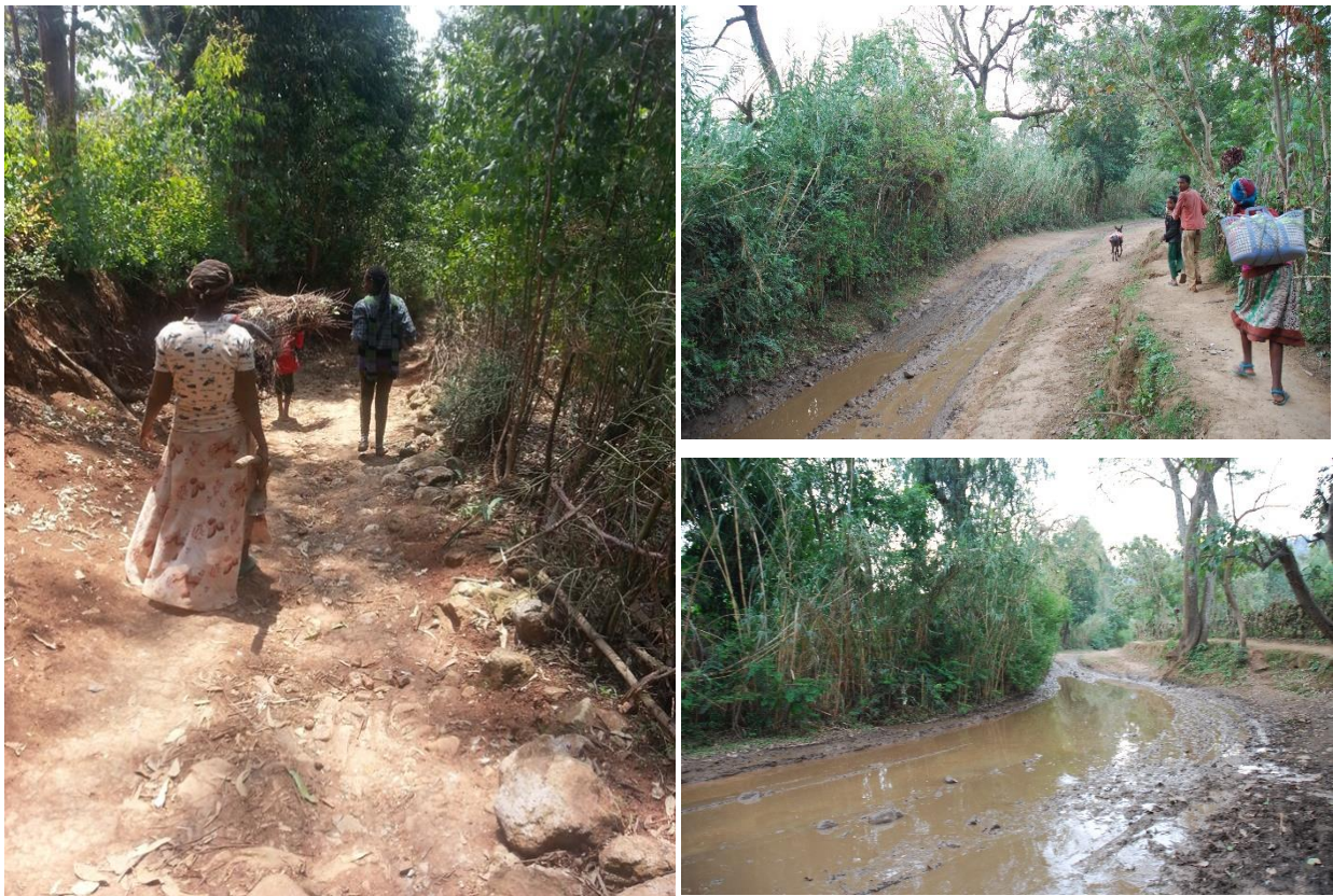
Photograph 13. Poor condition of roads in Aze Debo
