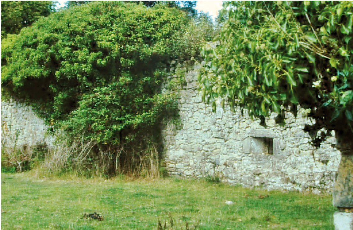
Fig. 2. Quarr Abbey, Isle of Wight. Wall and gun loops, 1365. Photo P. Purton.
