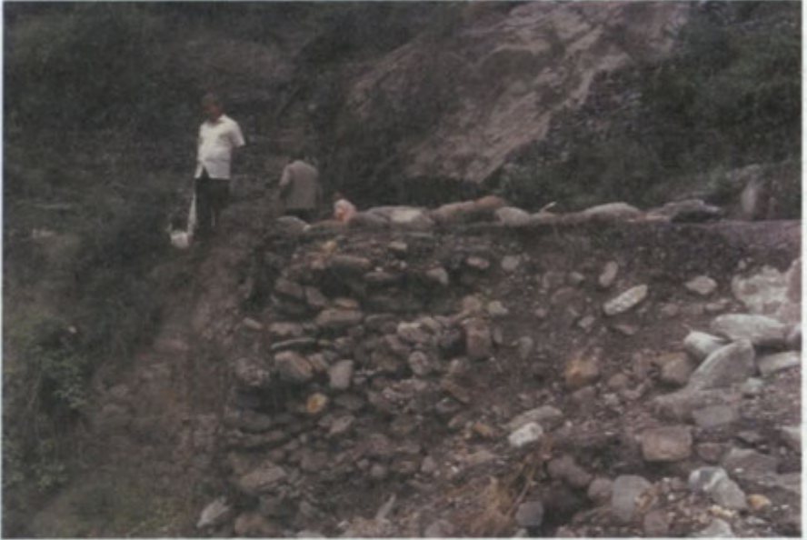
Highly denuded and subsiding Hill-Cart Road at lower Pagla jhora .
